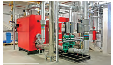
Hot water loop
